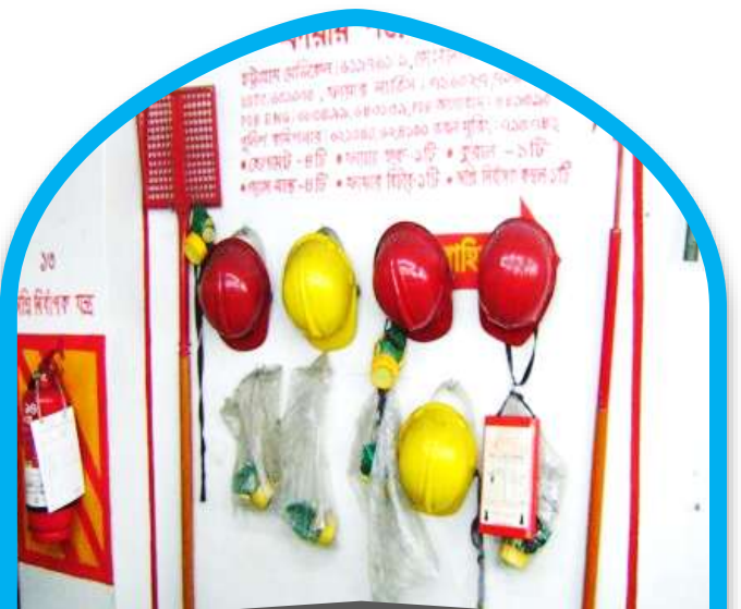
Fire Safety Equipment
